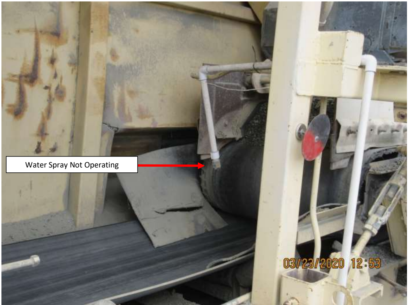
Photo 1 – Air Pollution Control Not in Operation
