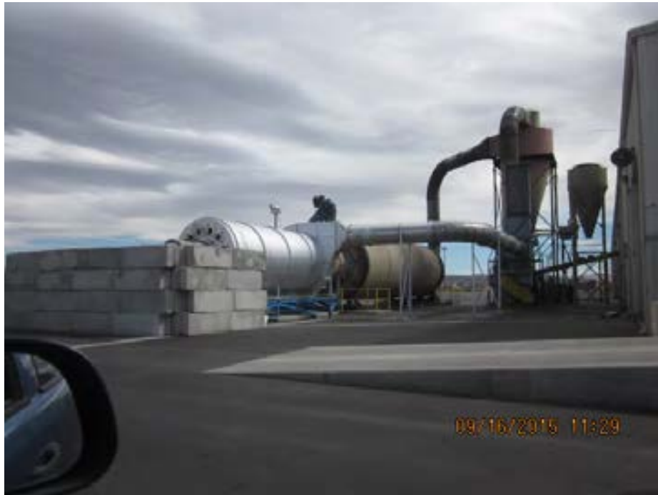
Photo 3: System 01 Natural Gas-Fired Burner (S2.001) and Drum Dryer.
